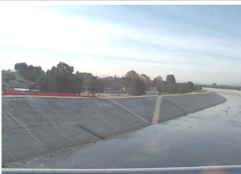
Left overbank protected by the Los Angeles River Levee near Rosecrans Boulevard
