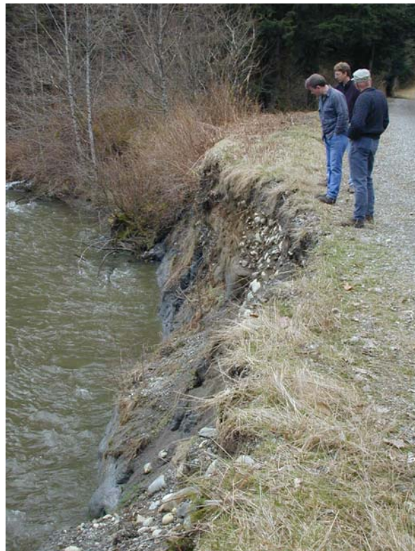
Forest road threatened by bank erosion along a bend of the Pilchuck River in Washington
